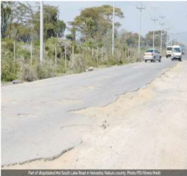
Part of dilapidated Moi South Lake Road in Naivasha, Nakuru county. Photo/PD/Wera Mwiti
